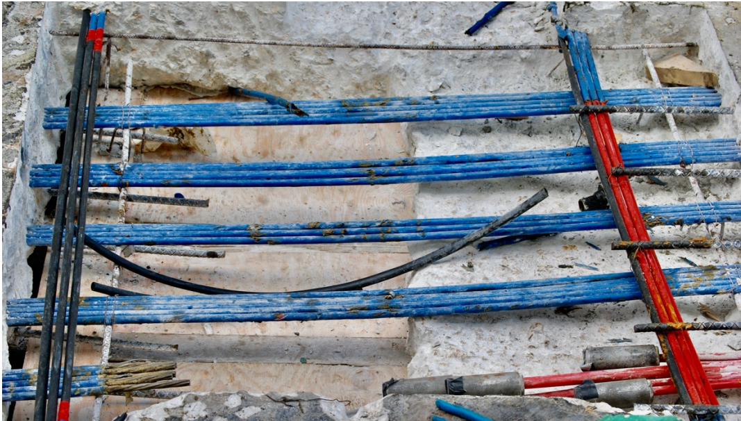
Photo: Groups of bundled tendons in a slab band line that is under repair.
